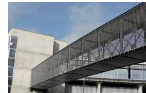
Robust safety with architectural mesh. Passerelle du Centre Balexert, Geneva, Switzerland.
