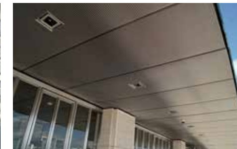
Ceiling made from framed mesh elements. Krasnodar, Stadium, Russia.
